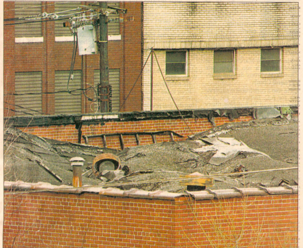
Run-down buildings are near collapse as rooftops begin to cave in around the city of Brownsville.
