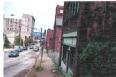
A Pittsburgh man is being fined $200 a day over this run-down building, one of many he owns in similar condition in downtown Brownsville. (SCOTT BEVERIDGE/O-R)
